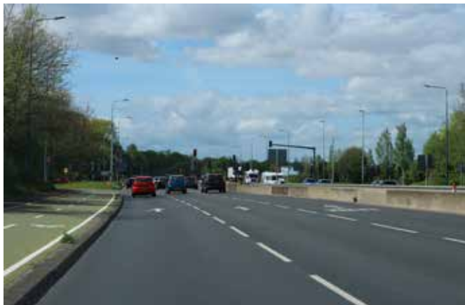
Concrete barriers preventing right turns at the Hambrook junction are being removed
